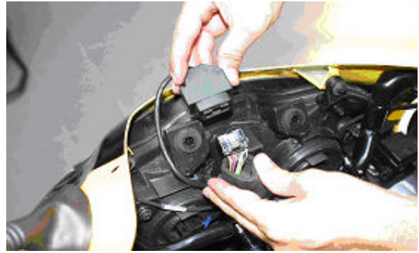
Figure 24 – wiring installation – particular of AMP connector.
